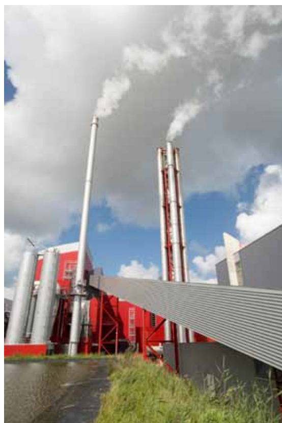
Photo 5 Medium-size power plant using waste wood in Alkmaar, the Netherlands (copyright M. Wijnbergh)
