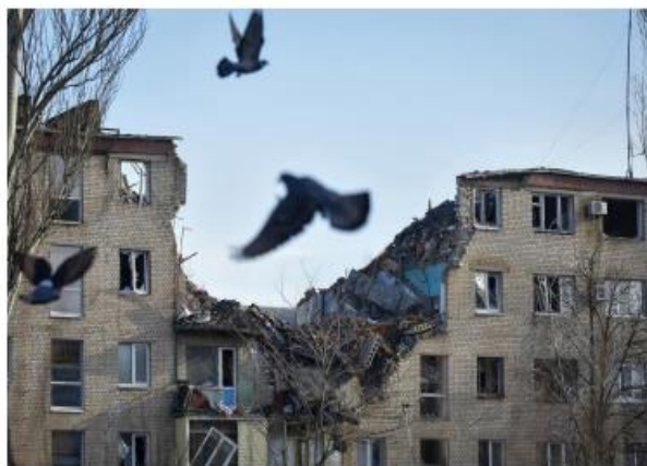
Building damaged by russian shells in Bakhmut
